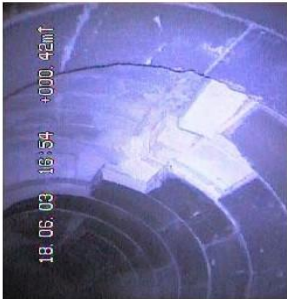
Fig. 7: Bricks Broken off the Refractory Lining in the Over Head Position of the Transfer Line
