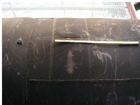
Fig. 5: Leakage and Bulging of the Transfer Line after a Short Term Overheating
