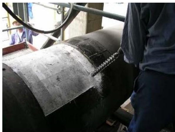
Fig. 6: Refractory after cutting away the Steel Shell
